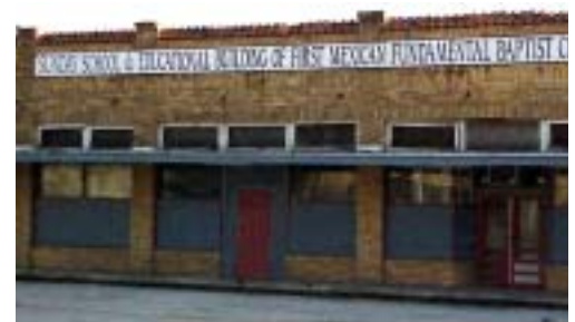
Non-conforming example of a commercial building that has window and door openings that have been partially covered with non-transparent materials
