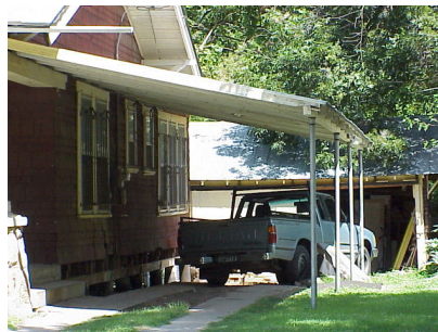
Non-conforming carport location and materials
