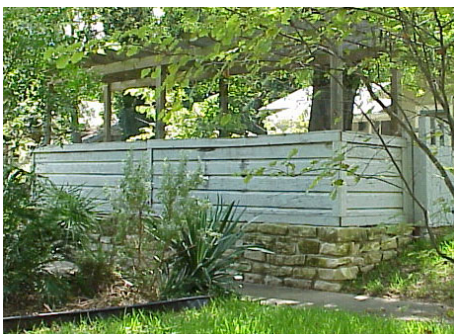
Example of non-conforming fencing (insufficient transparency)
