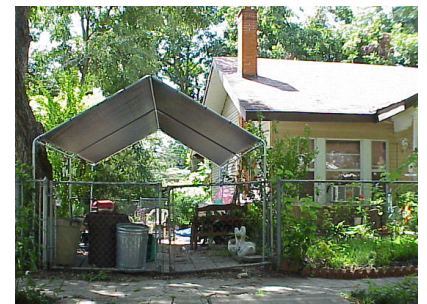
Non-conforming carport location and materials
